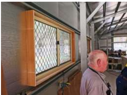
Once the internal wiring is roughed out, the walls will be lined with white Melamine
