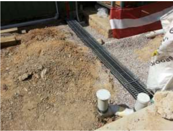
Channel drains installed with new sink connections for extension sink in foreground
